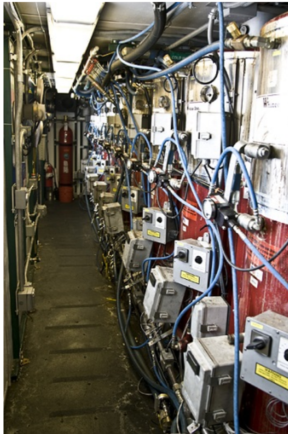
Figure 13: Model 75 heaters shown inside the Main Heating Plant
