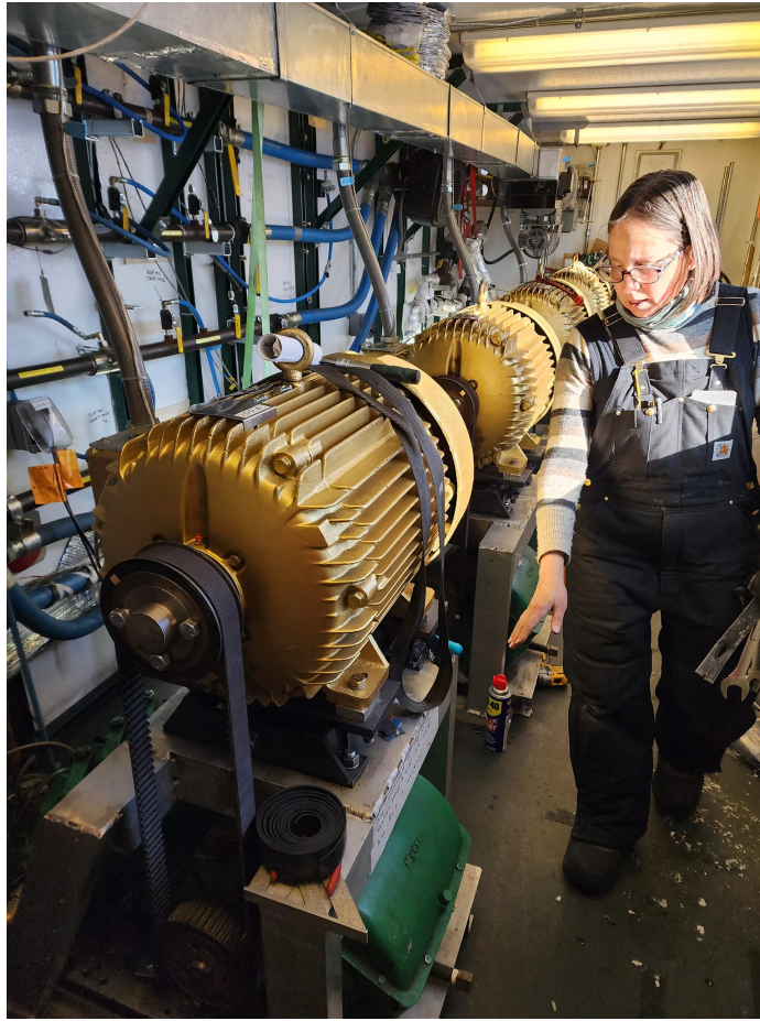
Figure 15: Four Myers pumps (green) and Baldor motors (gold) inside the High Pressure Pump building.
