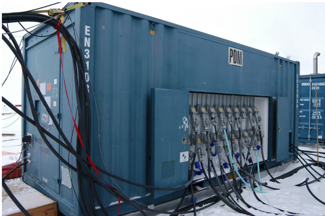
Figure 9: The Power Distribution Module distributes all of the electrical loads to the Seasonal Equipment Site and Tower Operations Site.
