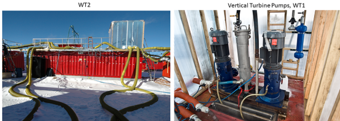
Figure 18: Left: Water Tank 2 at South Pole is shown in service during IceCube Gen1. Two of the existing water tanks will be repurposed for Gen2, and a third will be purchased to accommodate more water capacity than Gen1. Right: The “doghouse” structure on top of the water tank that shelters (from left to right) a vertical turbine pump, a bag filter, a vertical turbine pump, and a centrifugal pump.
